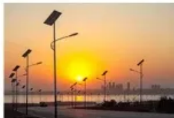
Solar Street Light
