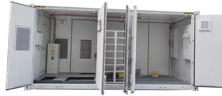
1075KW HH ESS
